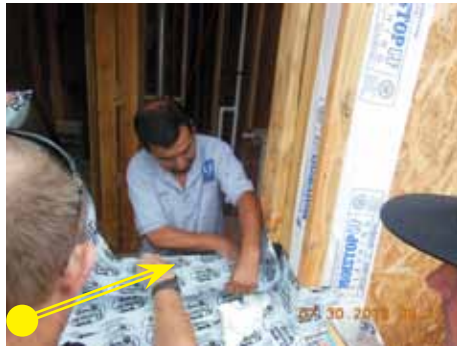
12. Apply Protecto wrap on to the framing sill and 6 inches up each trimmer.
