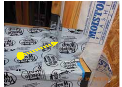
11. End dams cut and applied as shown. Use a 12" x 9" rectangular piece of Protecto Wrap as the end dam
