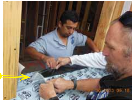
13. Apply Protecto wrap on to the framing sill and 6 inches up each trimmer.
