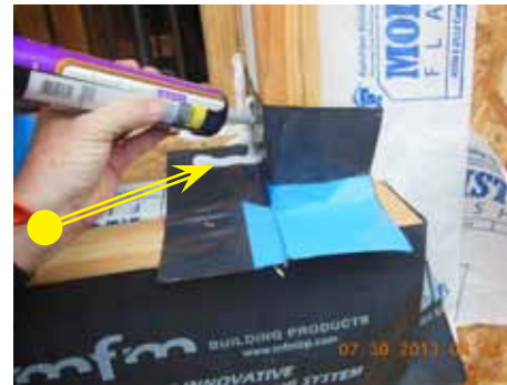
6. Sealant applied on top of GS 106 A flashing corner in preparation for GS 100 B corner
